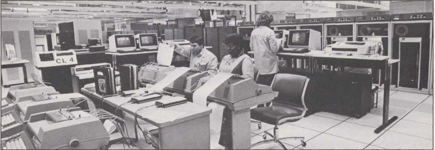
Equipment upgrades at the Brook Park Supercenter took place without disrupting operations.
