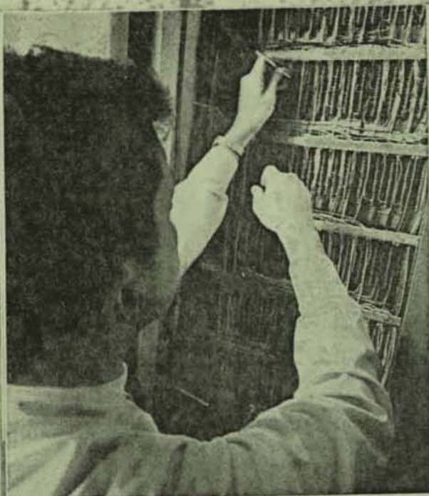
SUTHERLAND goes over the intricate wiring required to build ECHO. Each of four units has such a panel
