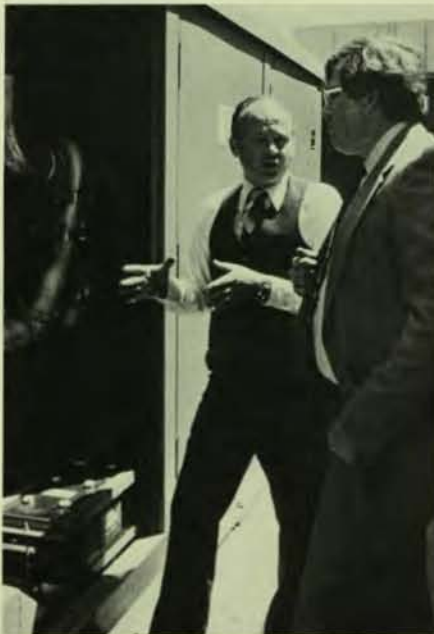
Gary, right, and Corporate Services Manager Russ Cooley inspect a new generator which can provide backup power for the company's central computer.
