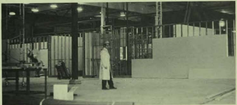
Phil Garcia surveys the progress of construction on the former fruit warehouse which is being transformed into one of the most modern semiconductor materials plants in the industry.
