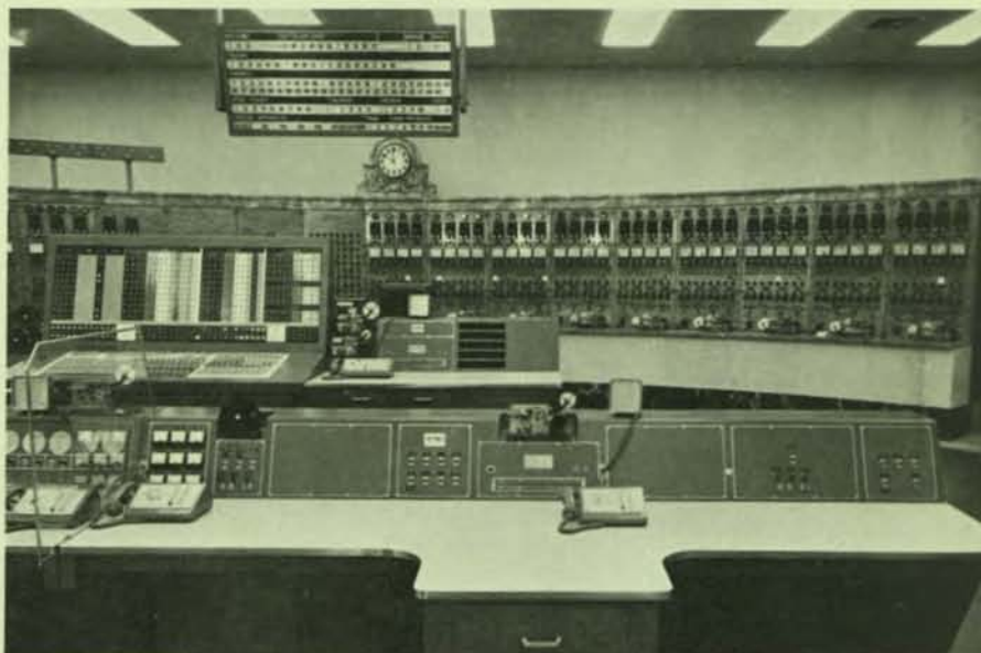
Part of the base station consoles for complete two-way mobile radio system installed by DuMont for the City of San Francisco Fire Department. This installation follows a similar complete system installed for the City's Police Department. Typical mobile unit installed in fire truck is shown at left.
