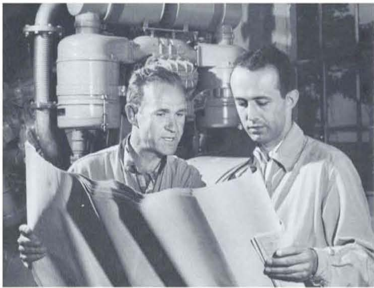
BACKBONE OF THE ISLAND: George Kovacs, Facilities Manager, shows the powerhouse setup to Leslie Moore, Hotel Manager.
