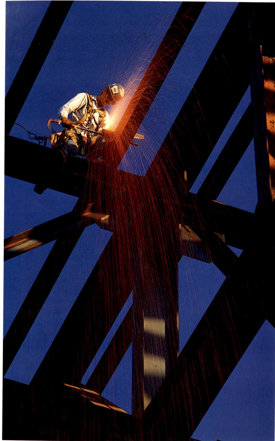
IN 1991, BOEING BEGAN CONSTRUCTION ON PLANT EXPANSIONS AND NEW FACILITIES THAT TOTAL SOME SEVEN MILLION SQUARE FEET. SHOWN HERE, A WELDER AT WORK ON GIRDERS FOR THE INTEGRATED AIRCRAFT SYSTEMS LABORATORY IN SEATTLE.
