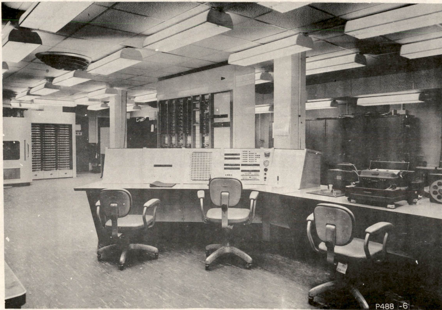
FIG. 1 TX-O COMPUTER ROOM
