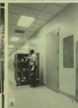
7. Facilities Manager Tom Ellerbee checks the system that brings gases, de-smogged air into areas of the building through pipes housed in a 10-foot section between floors.
