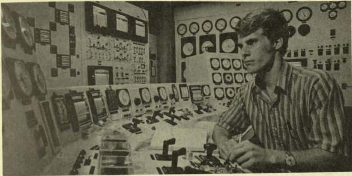
Control room operator, Humboldt Bay Nuclear Power Plant.
