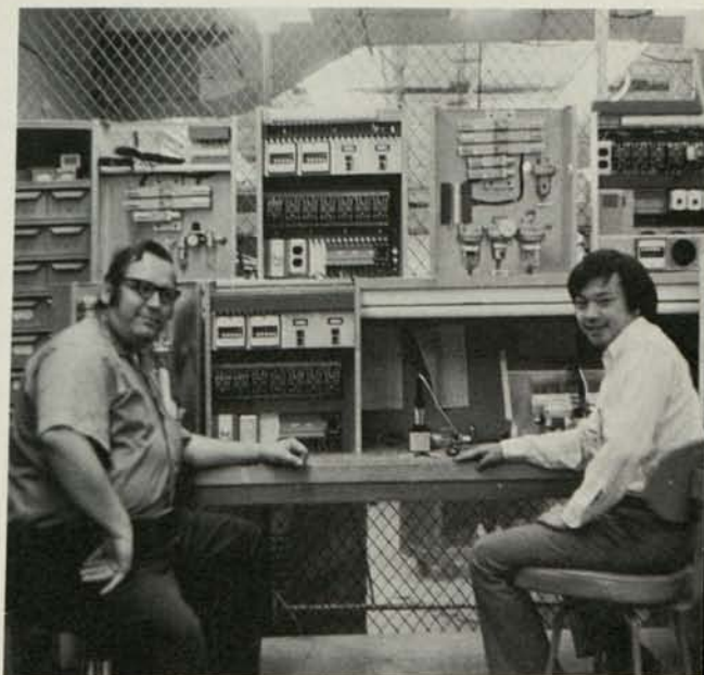
Marlow Stephens (left), supervisor of the electrical shop; and Chris Chen, electrical technician; pose next to the control panels they devised for the new equipment for Healdsburg.
