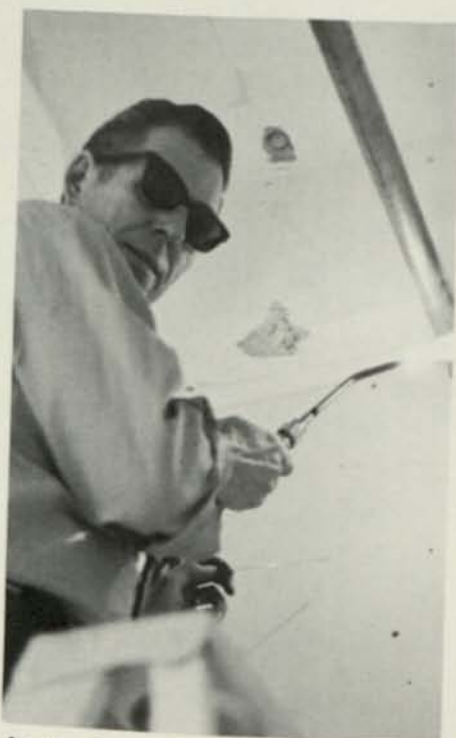
In the basement of Building 3, Don King, plumber, is welding a plumbing line which runs through the new lap-ping area.
